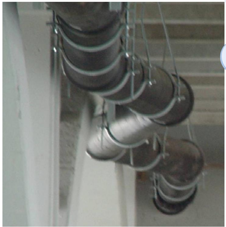
Pipeline “Snaking” Due to Inadequate Lateral Support
